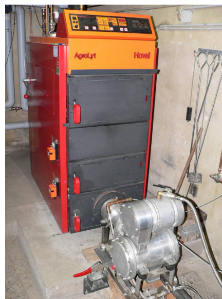
Abb. 2 Biomassekessel/ Stirling Kombination, in Sulzbach
