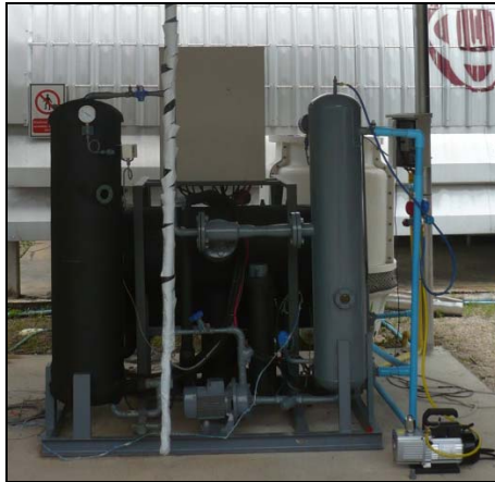
Fig 2. Solar-Driven 1 Ton Single-Stage Steam Refrigeration System with a 2.40 m 2 roof-mounted Heat-pipe Evacuated Tube Collector
